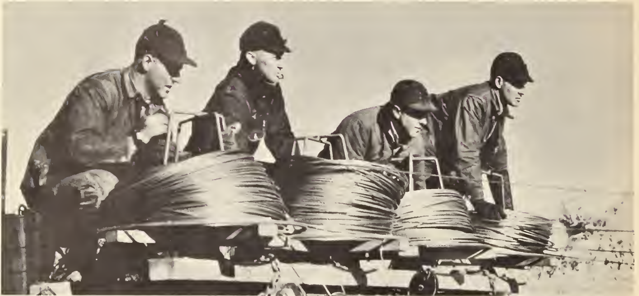
Crew stringing line covered several miles a day. A crew followed to take the line up to the top of the poles.
